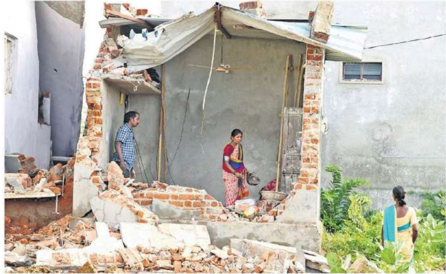
A woman searches for her belongings amid the rubble following demolition of houses in Mahabubnagar on Friday.
