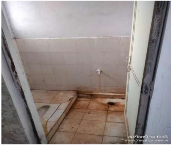
Photograph 21: Washrooms, Dindori, MP
