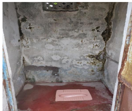
Washroom in KGBV-H with no doors and water flush system
